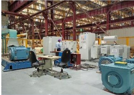
Traction Motor Testing facility
