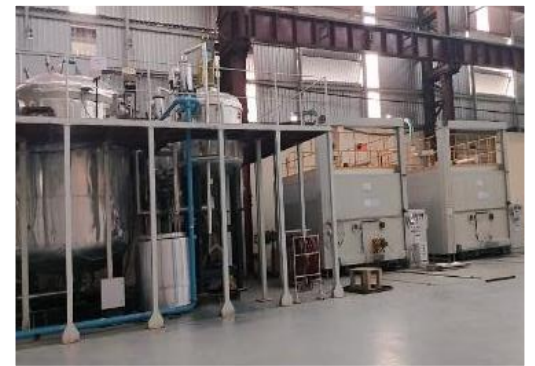
VPI Plant with Oven
