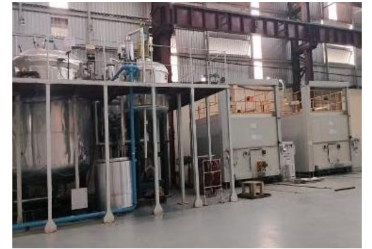
VPI Plant with Oven
